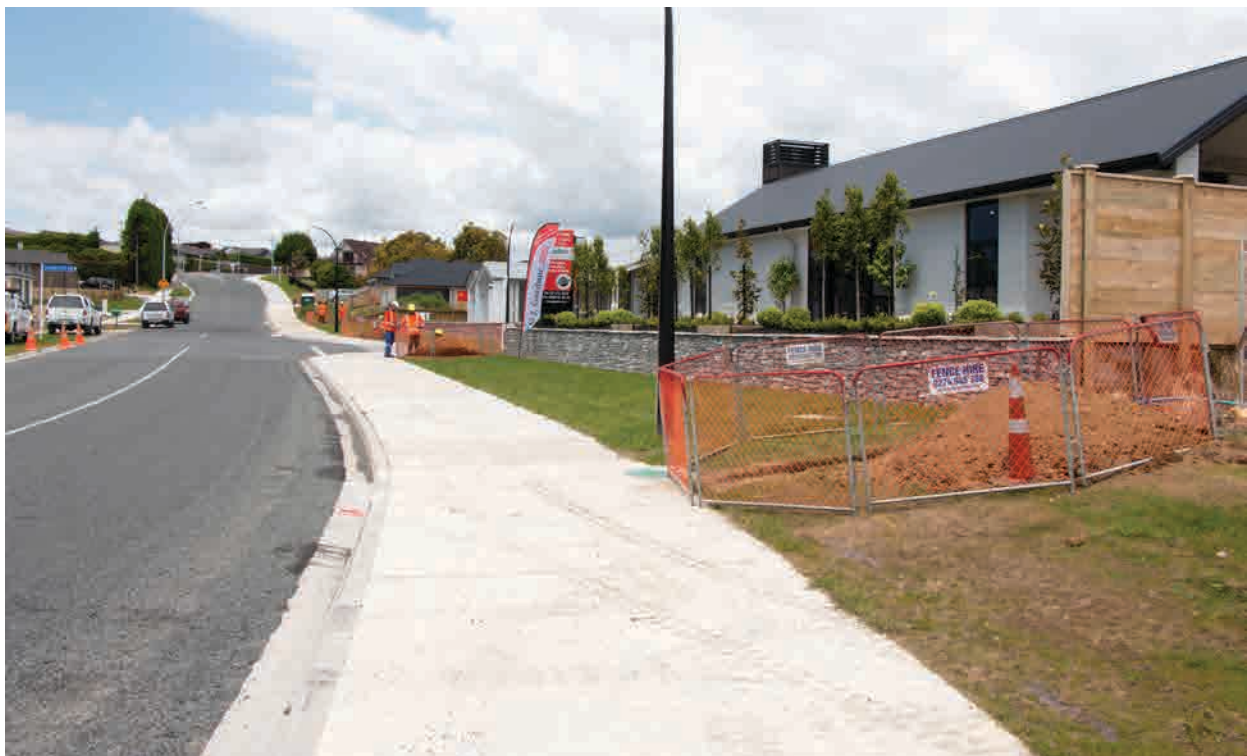
Figure 3. Kaylene Place showing lateral potholes to expose existing services prior to a drill shot.
